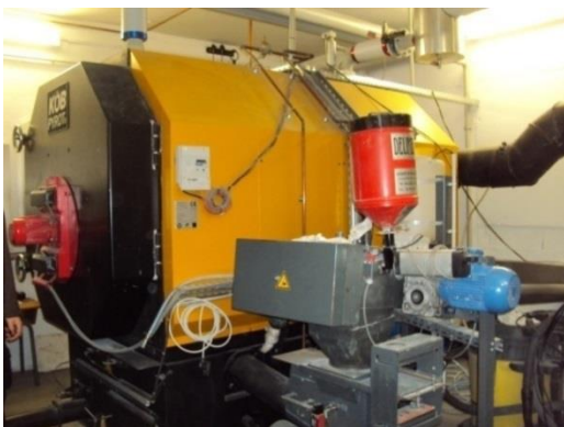
Chaudière poly combustible - CRAP
